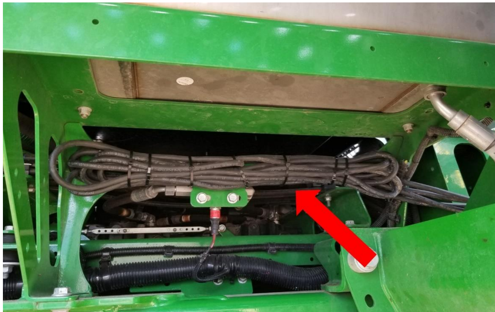
Fig. 19: Power Cable Bundled & Secured to Frame Under Sprayer Cab
